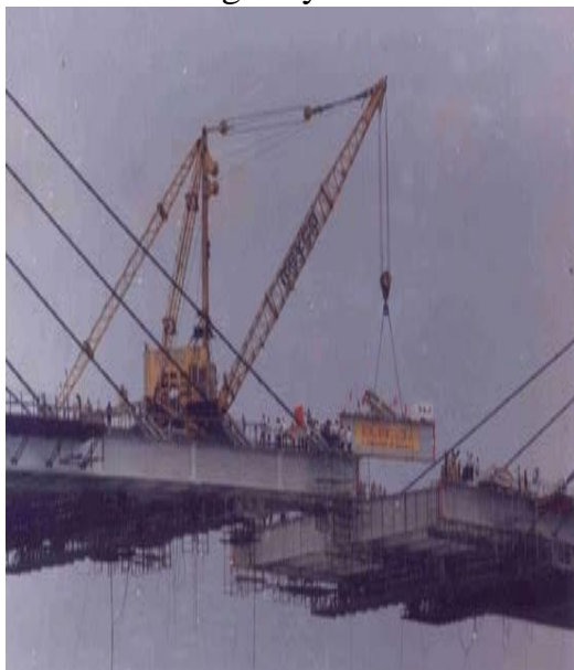
Figure 4. The mid-portion of the deck of the Second Hooghly Bridge being constructed, vividly showing some of the high capacity cranes used
